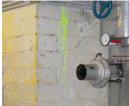
Detection of a leaky water-carrying pipe in a building by passing in uranine and performing a subsequent UV inspection.
