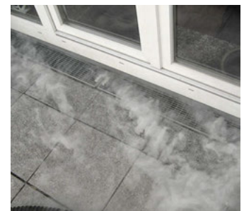
Defective sealing of a roof-top terrace.
